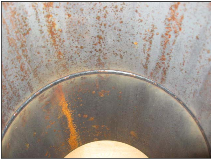
Figure 16. Photograph of the inside of the same hybrid pipe weld, illustrating the consistent reinforcement along the inside diameter.
