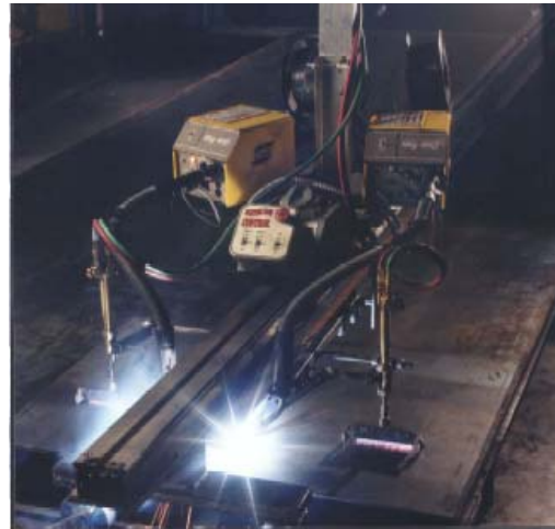
Heating during welding can help balance the welding-induced compressive stresses in thin plate structures.
