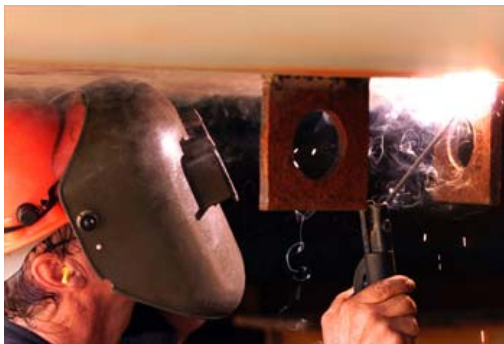
The ultra-light GMAW-P welder will replace Shielded Metal Arc or "stick" welding in many outfitting applications.
